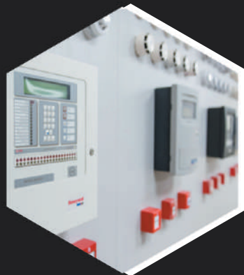
Building Management Systems - Access Controls, Fire Alarm, Automation Etc.
