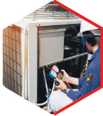
HVAC (Operation & Maintenance)
